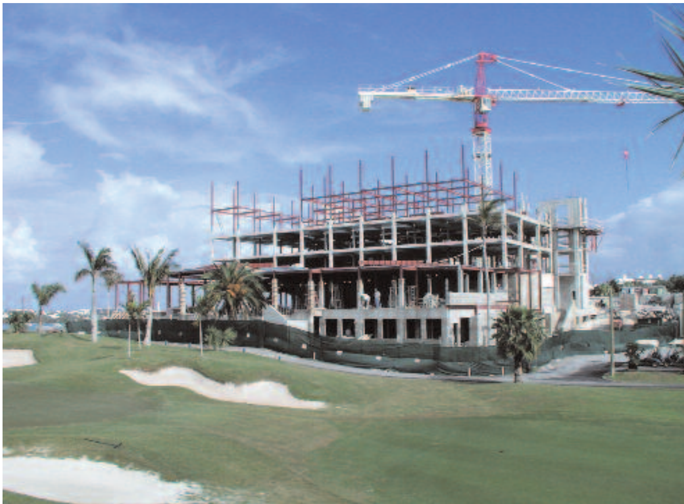
Although some of the old structural steel was perfect, major changes had to be made to create top-class apartments
